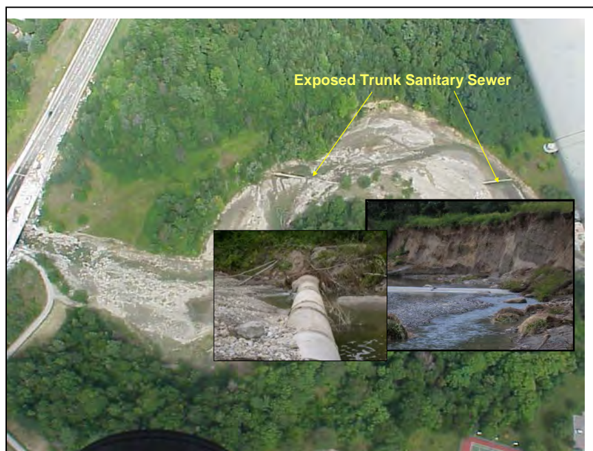
Figure E6-9: Picture and Location of STS erosion in Highland Creek watershed caused by Aug 19th, 2005 storm extreme weather event
