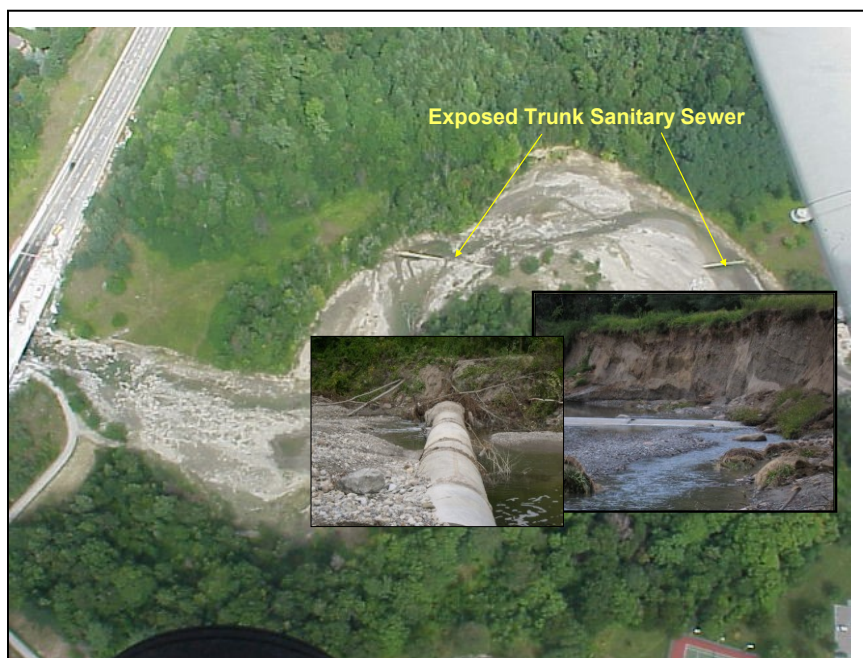
Figure E2.9: Picture and Location of STS Erosion in Highland Creek watershed caused by Aug 19th, 2005 Storm Extreme Weather Event
